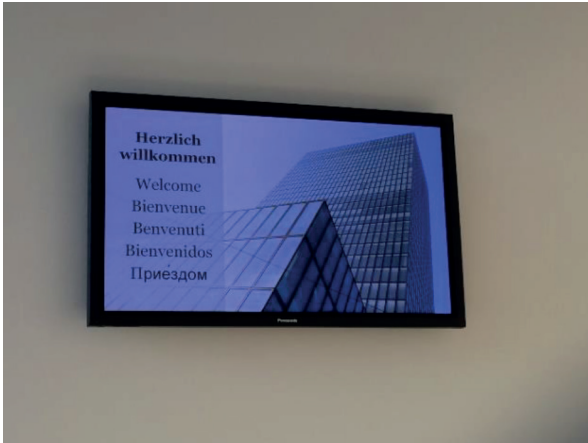
65» PLASMA SCREEN IN THE ENTRANCE AREA/ESCALATOR
